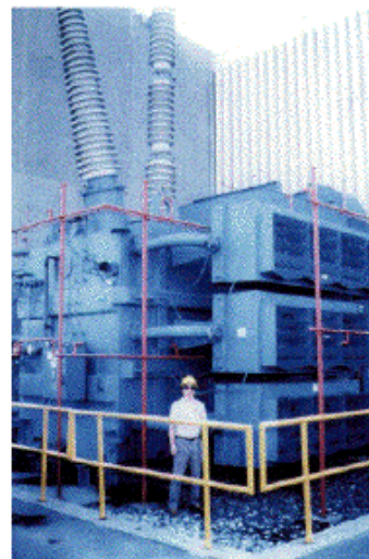
PJM Public Service Step Up Transformer
